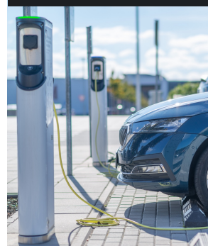
EV Car Charging
